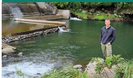
New Taranaki field officer Jack Harland at Manawa Energy's Motukawa hydro diversion weir and fish pass on the Manganui River.
