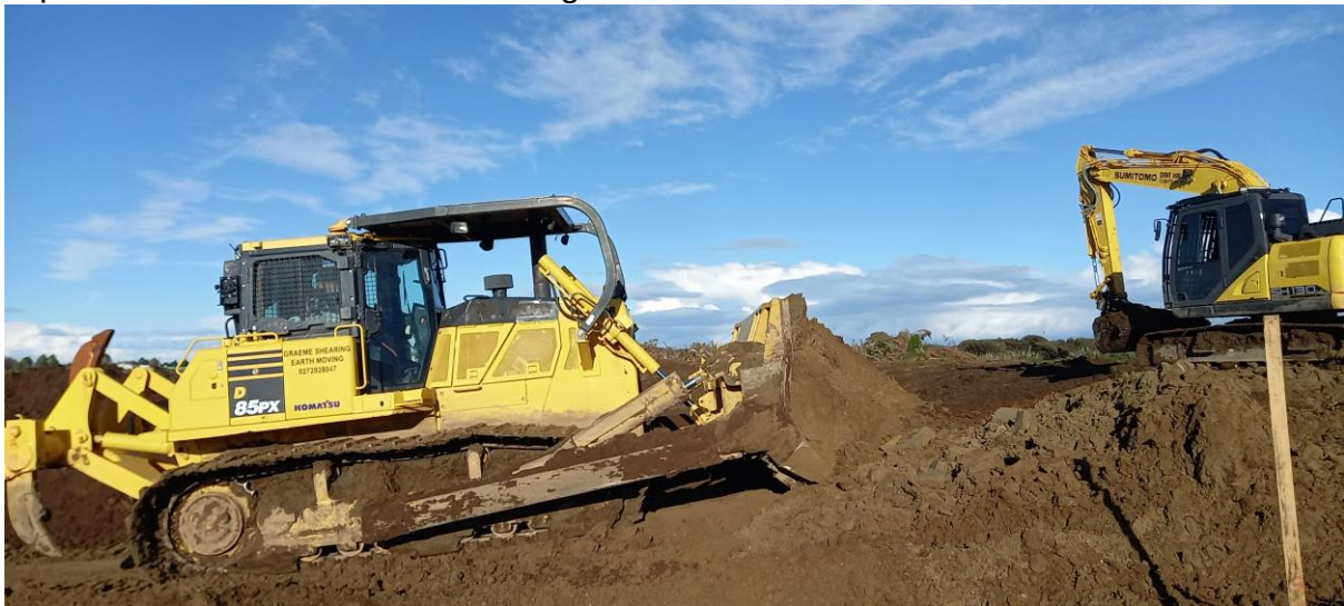
Dozer and digger working in combination to construct dam for Eastern Wetland.
