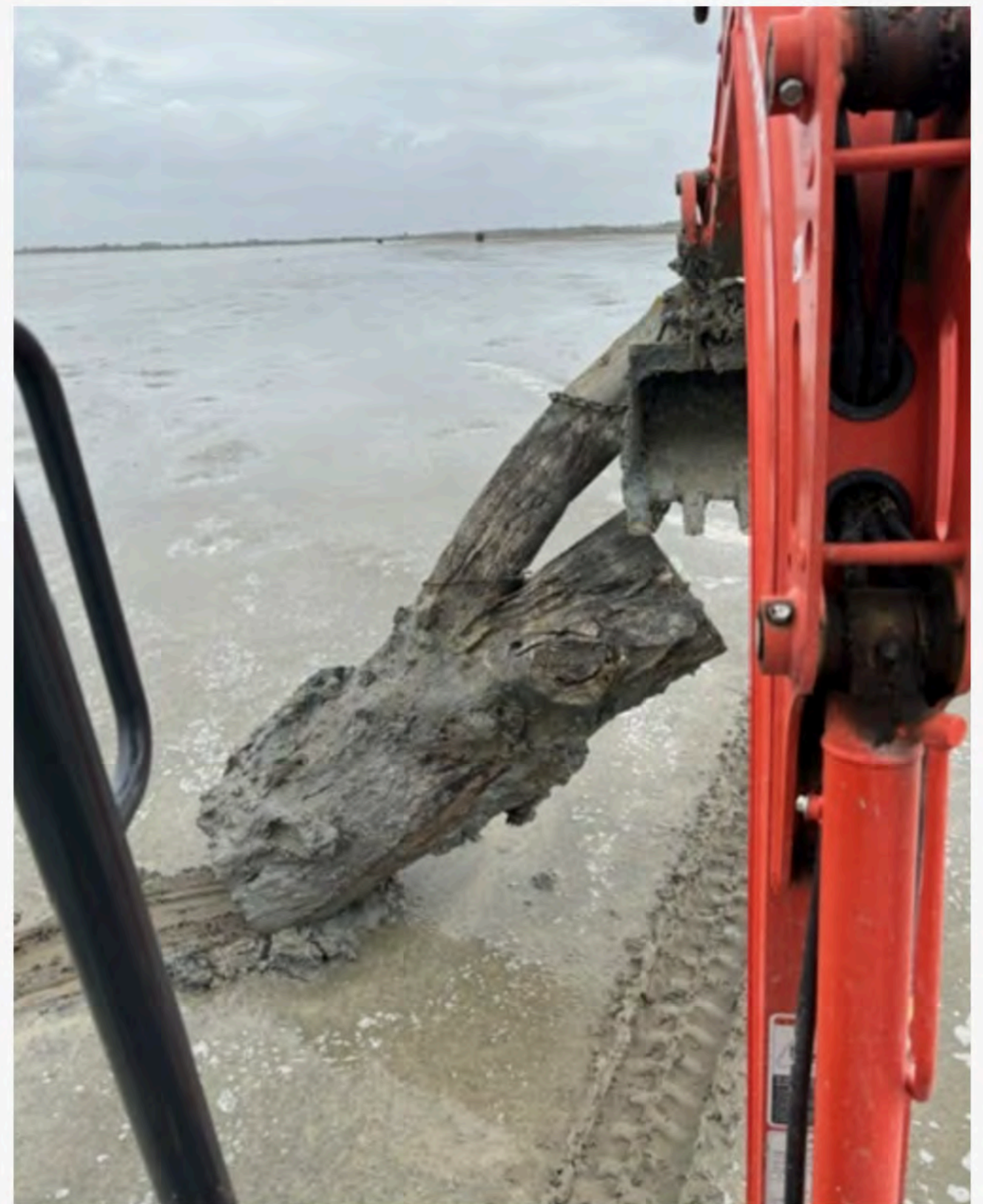
Hazardous tree stump being removed.
