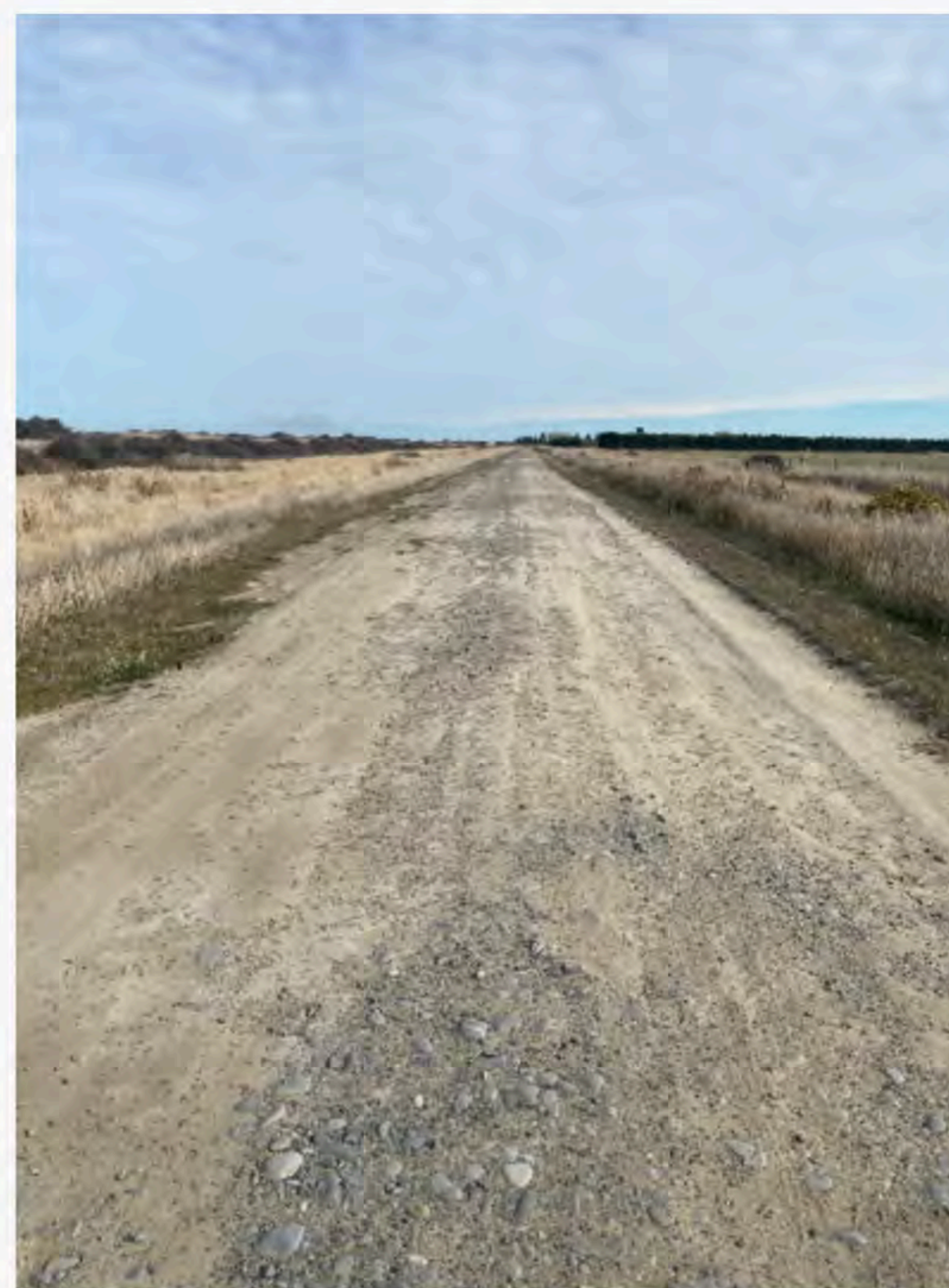
Section of the unformed legal road to the Halswell boat ramp that still needs to be graveled.
