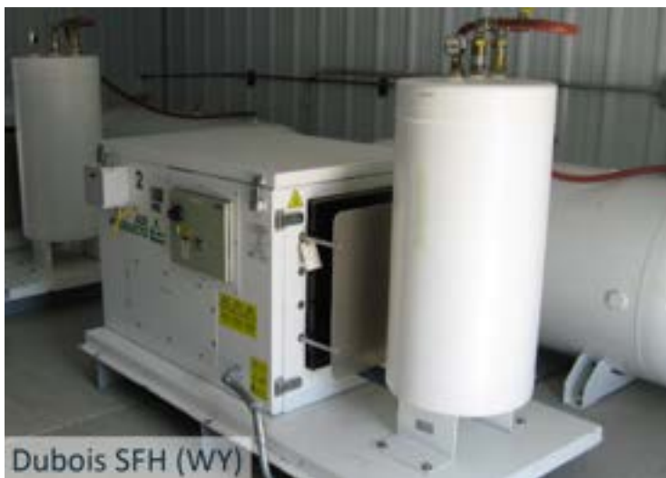
Pressure swing absorption unit
