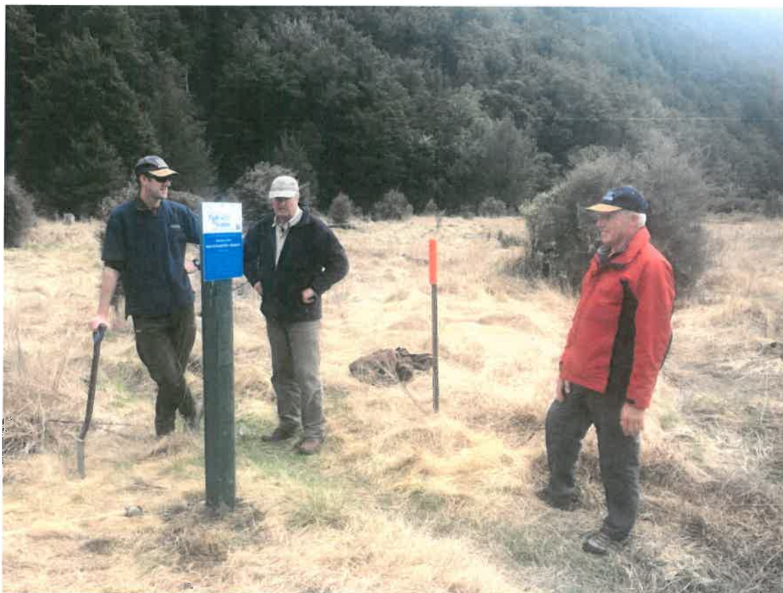
Travers River signage installation for one of Nelson/Marlborough's first two designated back country fisheries (staff member and 2 Councillors in the shot).
